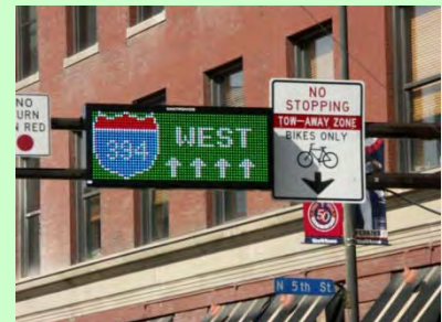
Variable Message Sign in Minneapolis
